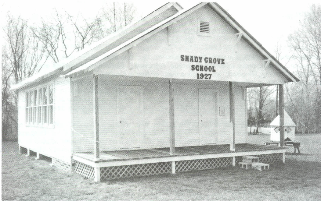
The Shady Grove School renovation is rapidly coming together. Porch has just been decked With timbers removed from the West Side of Square demolition. The Bell Tower has been installed.
