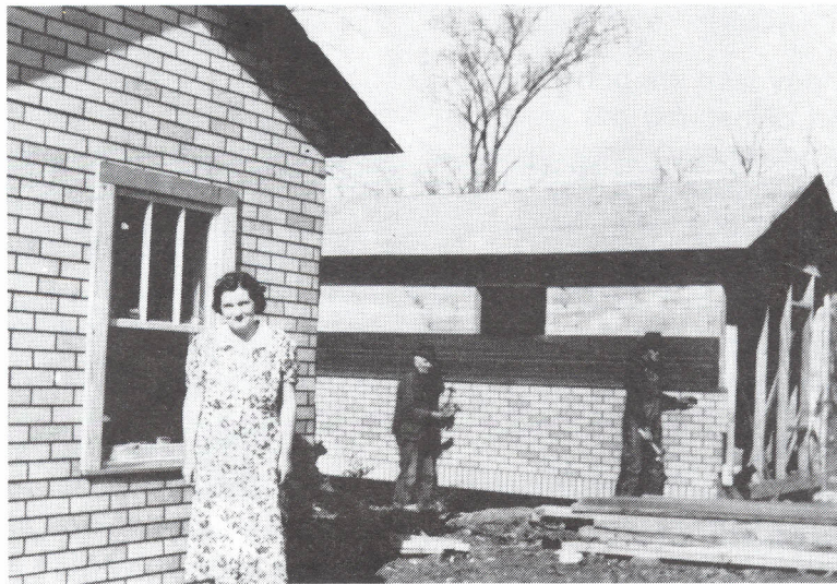
Constructing cabins at Spencer. Elizabeth Spencer in front of 1st cabin built
